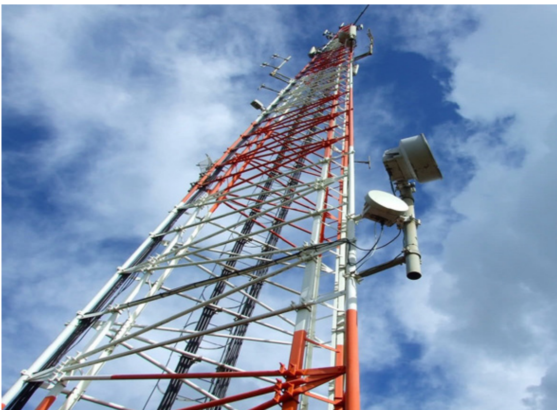
Improved telecommunications infrastructure.
