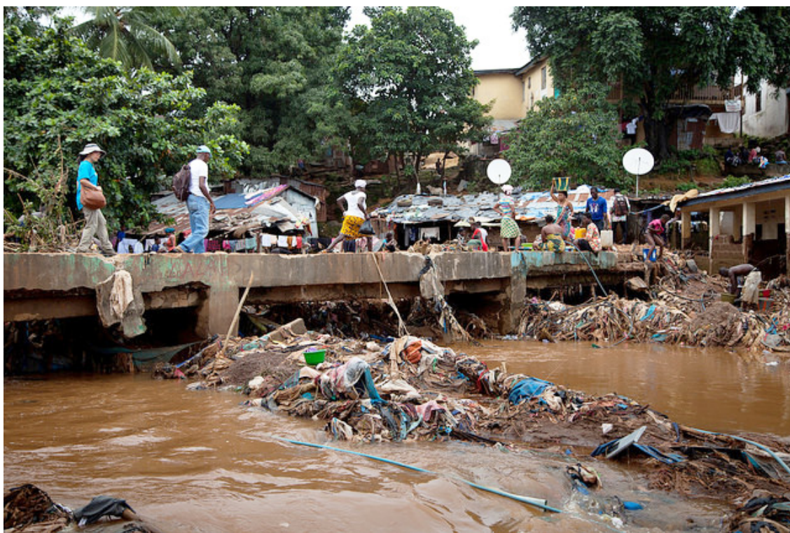
Indiscriminately dumped garbage and poor drainage systems.
